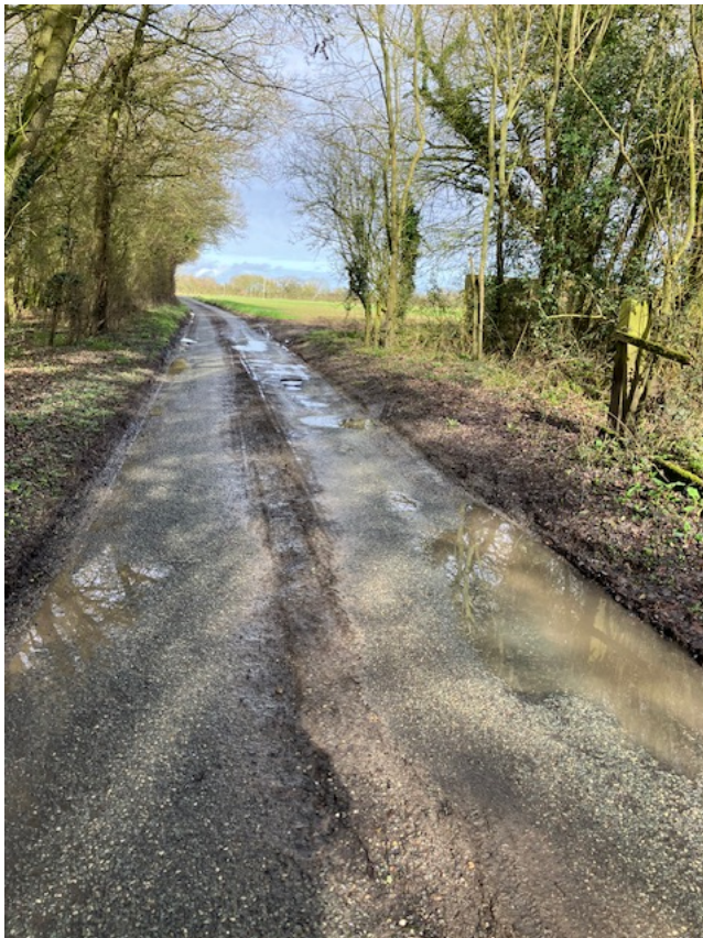
Shotesham Road in Woodton showing the unsuitability of these lanes for HGV traffic.
